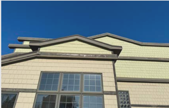
13 - Exterior Envelope - Missing Trim
