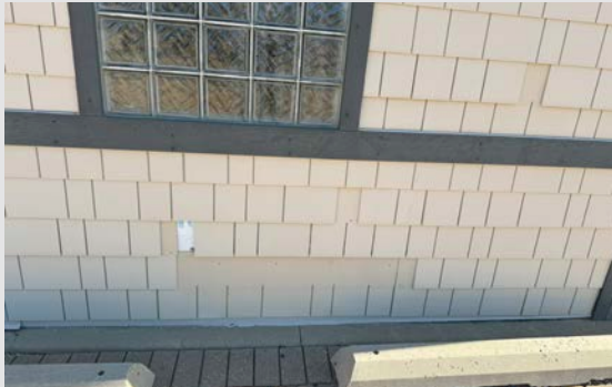
10 - Exterior Envelope - Missing Siding
